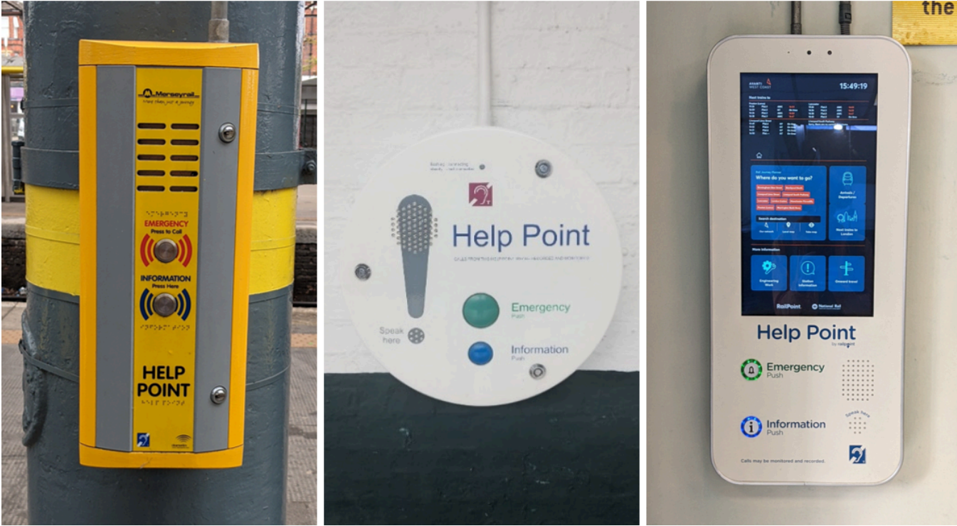
Figure 1.1 Examples of help points, left to right: Southport (Merseyrail), Cheltenham Spa (Great Western Railway) and Wigan North Western (Avanti West Coast)
