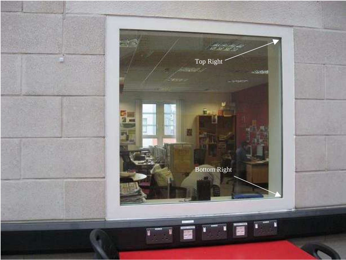
Figure 25 Room 1.15 Window. Corners of glass pane.
