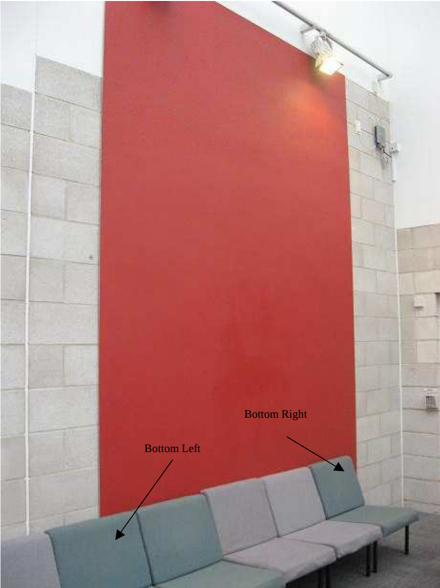
Figure 28 Features on Red Panel on upper floor by Room 2.16 door. The two bottom corners (not visible in the picture).
