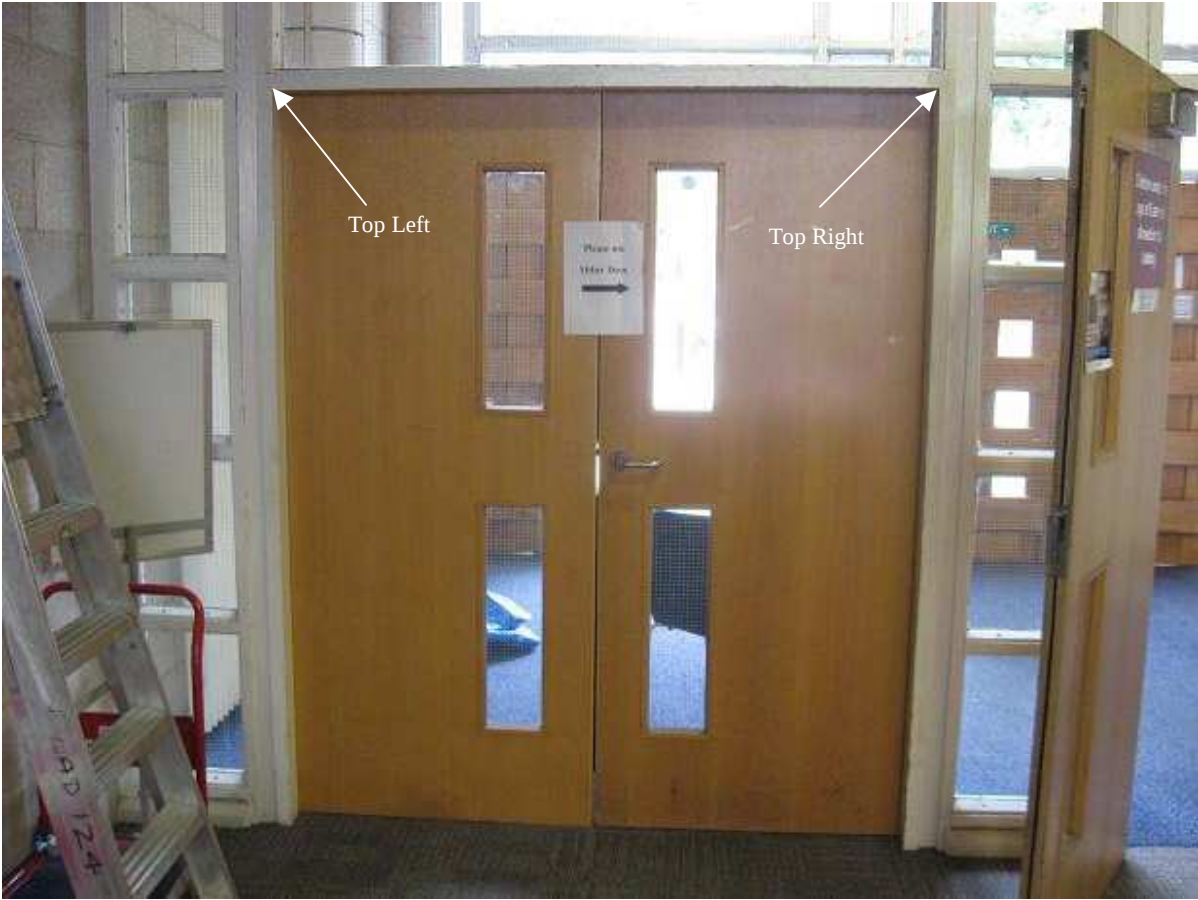
Figure 31 Features on Main Entrance Inner Left Door.
