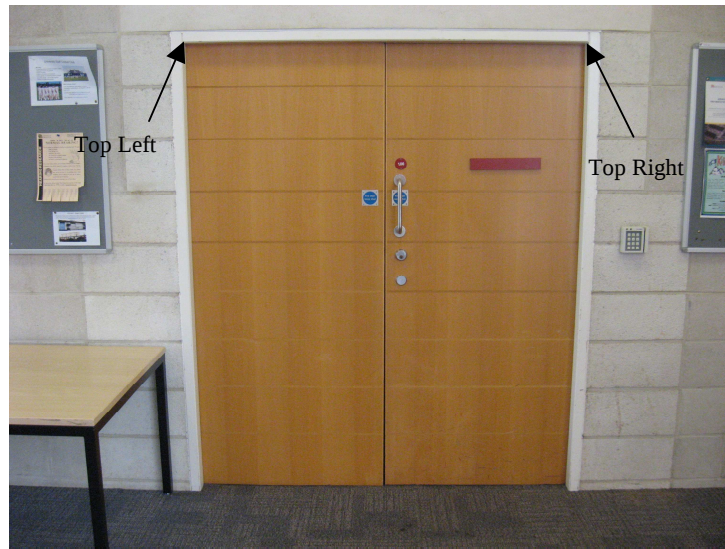
Figure 18 Features round Room 1.06 door. Outside corners of wooden frame.
