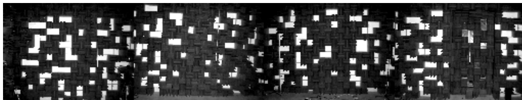
Figure 12. Panoramic composite view of walls with 336 wedges removed
