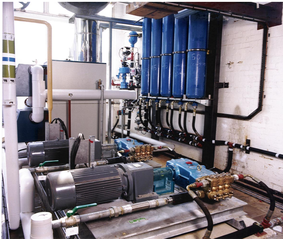
Figure 2.4: High pressure plant equipment.
